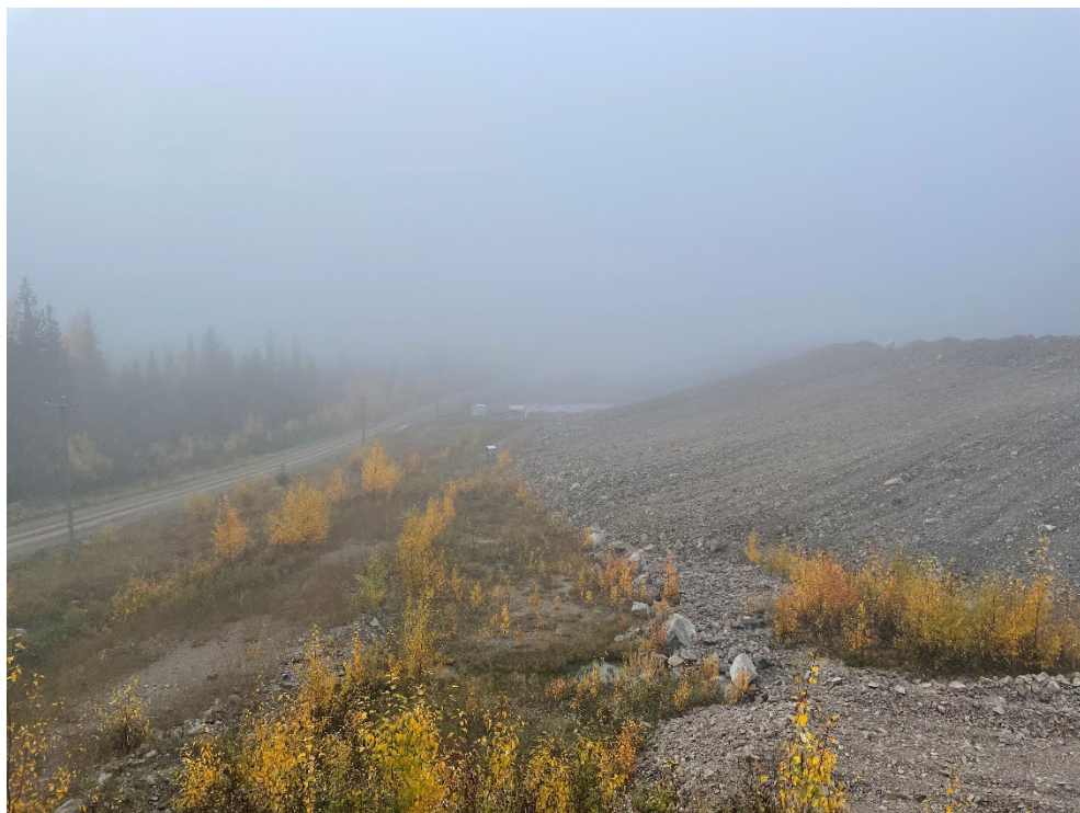
Photo 5: View Southwest Through the Southeast Tailings Storage Facility (TSF) Foundation Preparation Area
