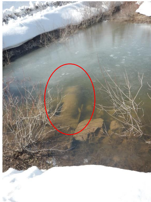
Figure 11 March 29, 2023. Upper Long Ditch Sump with primary pipeline submerged. The pipeline is frozen and not conveying water.
