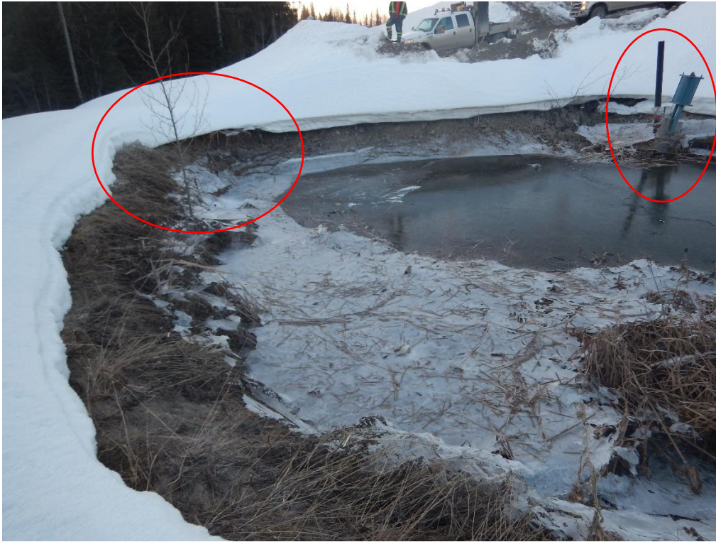
Figure 6 March 28, 2023. The Lower Long Ditch Sump showing discharge channel under snow in upper left and partially closed knife gate in upper right after incident. Note high water mark shown by ice level.
