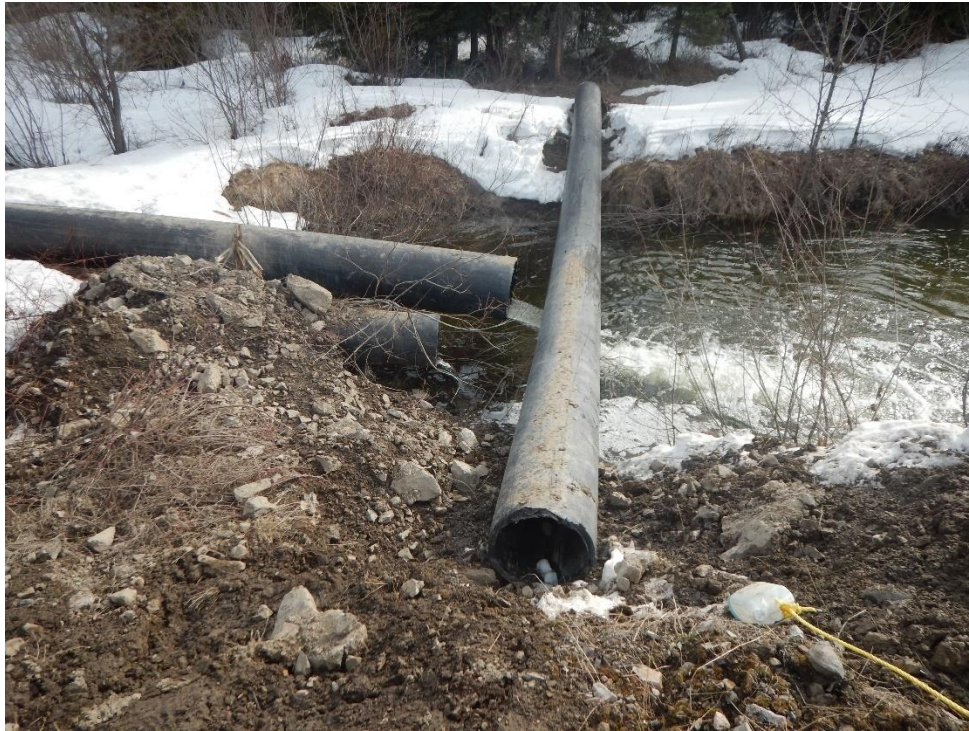
Figure 16 March 11, 2023. Primary Long Ditch Pipeline operating as intended and discharging downstream. The pipe across the ditch was used to insert steam apparatus into frozen pipe and is not part of the collection system.
