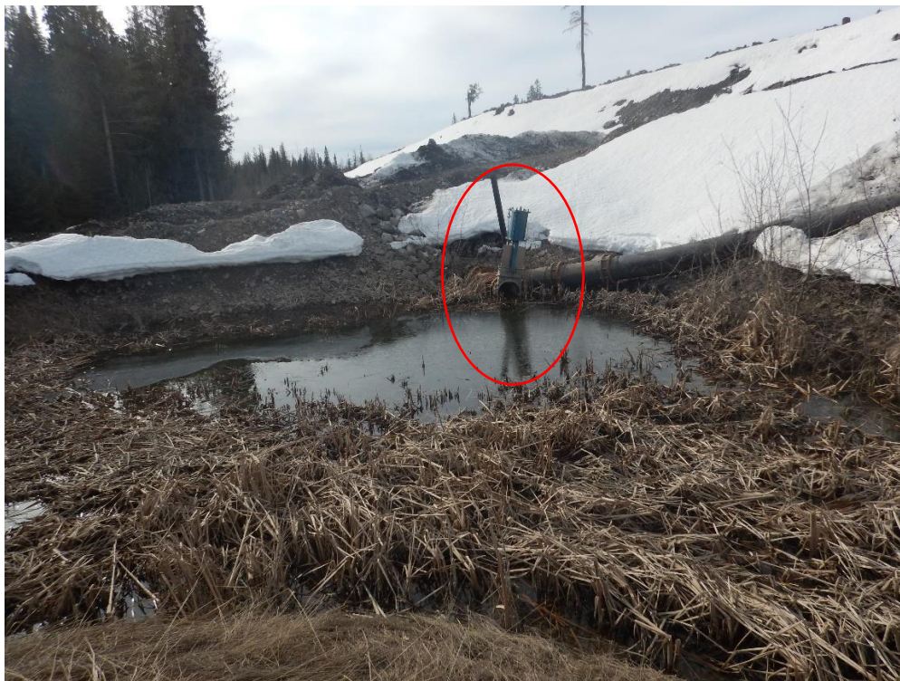
Figure 7 March 28, 2023. Lower Long Ditch Sump with knife gate opened.
