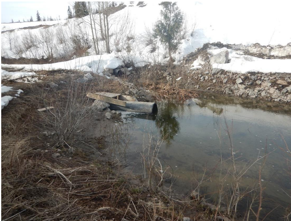
Figure 15 March 11, 2023. Primary Long Ditch Pipeline operating as intended.
