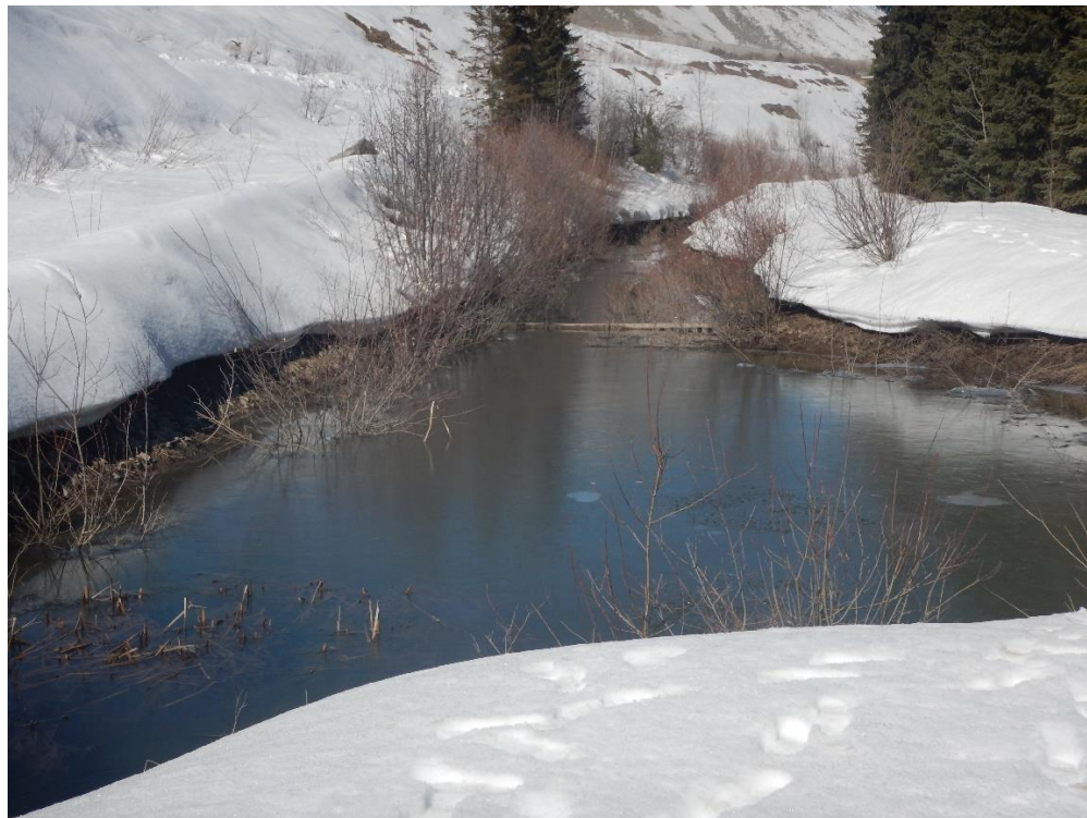
Figure 9 March 28, 2023. Upper Long Ditch Sump inundated with primary pipeline submerged. Discharge to lower sump occurring in lower left.
